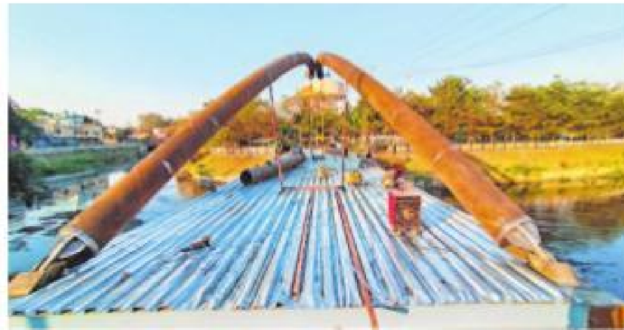
Construction work in full swing at the site on Friday Pic by ANAND SHIVRE
